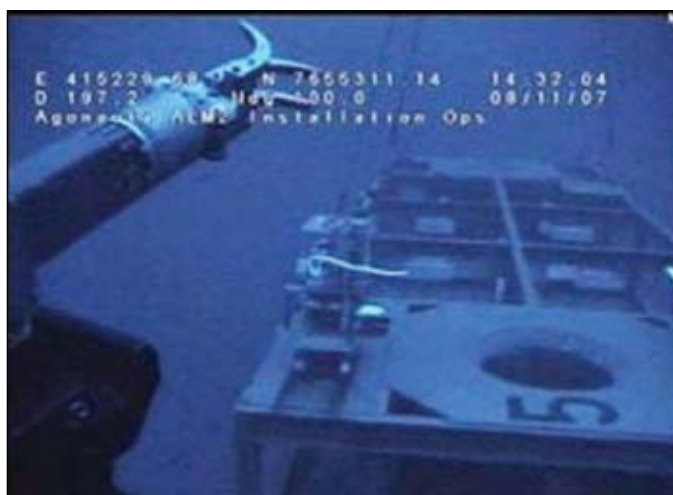
The base of the ALM2 is installed at Argonauta field in August 2007 (Fig. 5; photo from Shell).
